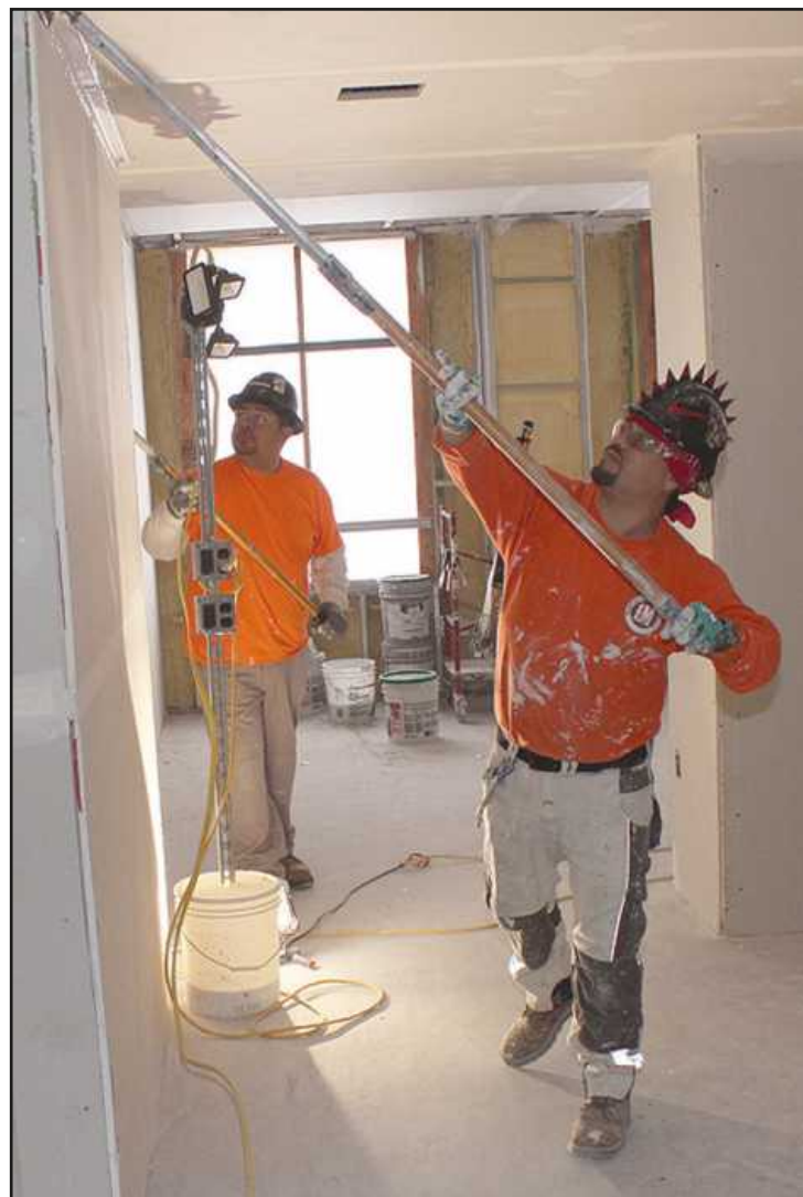
FINISHING DRYWALL on the 13th floor of the Residences @ 150 Bagley project are (l-r) Jose Alfredo and Hamlet Martinez of Michigan Painters District Council 1M. They're employed by the Brinker Team.
