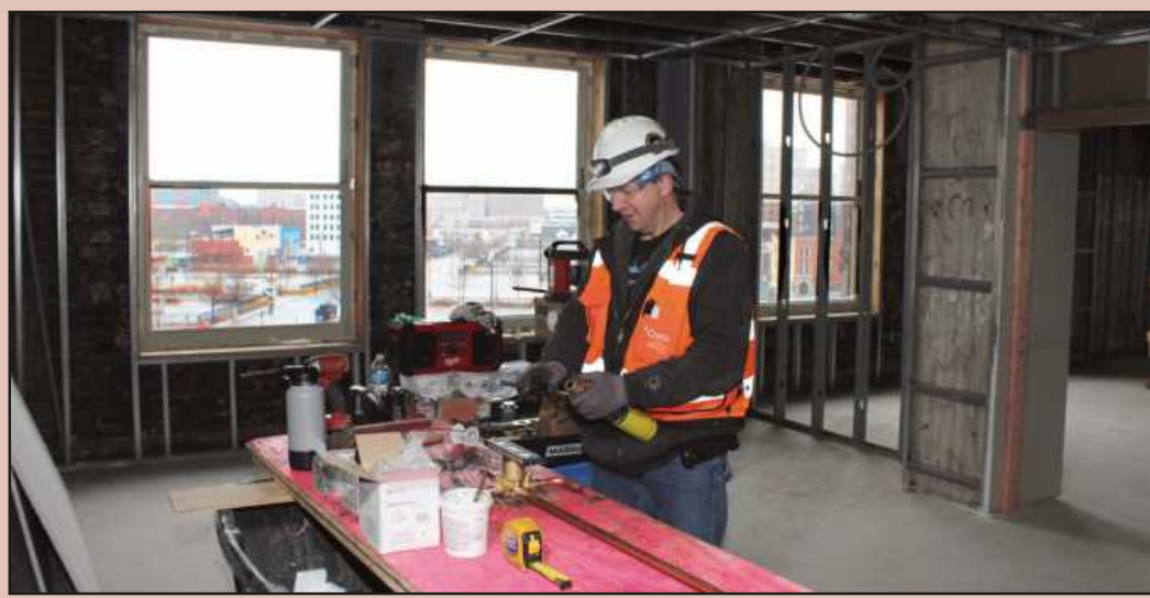
SOLDERING A SHOWER VALVE in what will be a fifth-floor apartment at the 150 Bagley project in Detroit is Randall Meyer of Plumbers Local 98. He's employed by Ben Washington and Sons Plumbing and Heating. Photo credits: Marty Mulcahy
