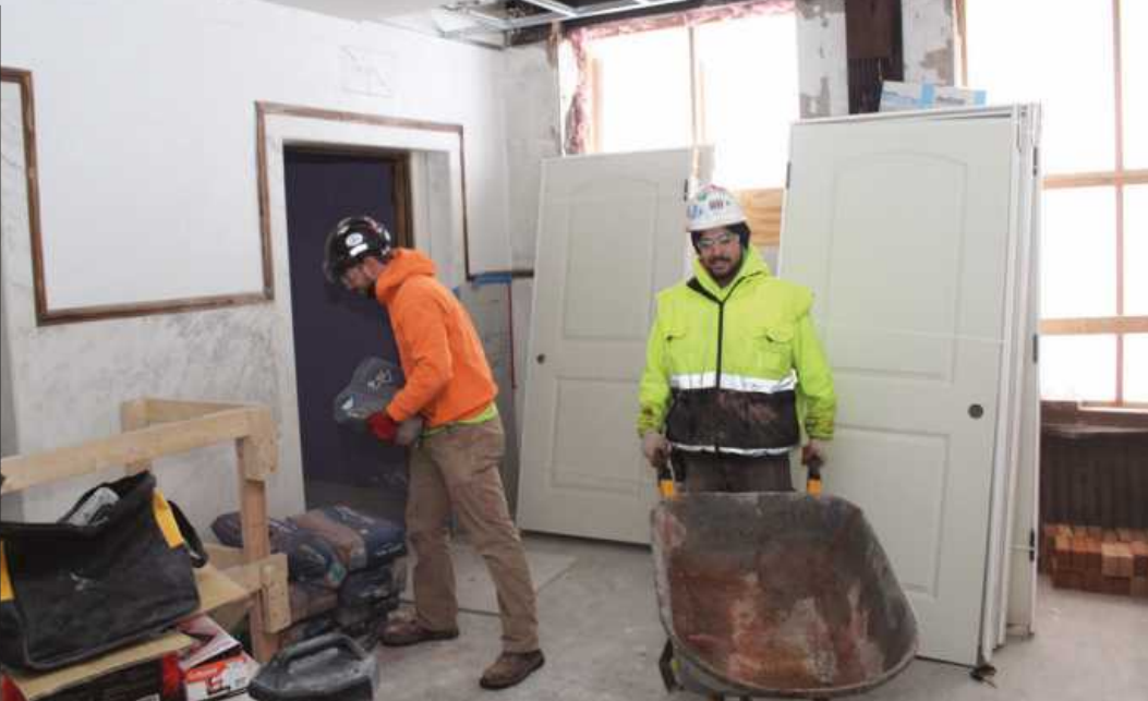
MOVING MORTAR on the 17th floor of the Residences @ 150 Bagley project in Detroit are (l-r) masons Cylar Rea and Mohamed Haimed of Bricklayers and Allied Craftworkers Local 2. They're employed by Leidal and Hart.
