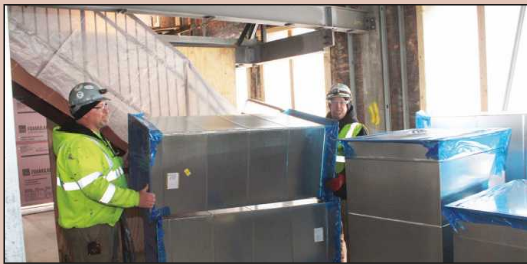
SETTING DUCTWORK on the 18th floor of the 150 Bagley project in Detroit are (l-r) Eric Allen and Dan Quinn, Sr. of Sheet Metal Workers Local 80. They're employed by Sylvan Inc.
