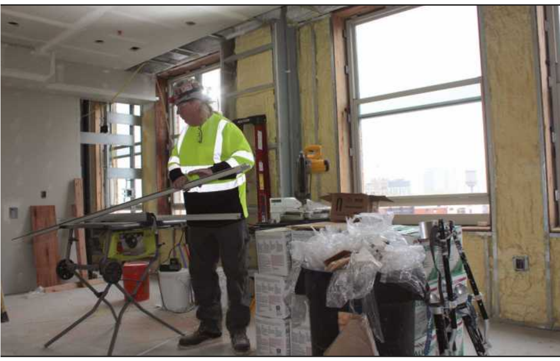
CUTTING WINDOW FRAMES at the Residences @ 150 Bagley project in Detroit is Mike Kehoe of Glaziers and Glassworkers Local 357. He's employed by Modern Mirror.
