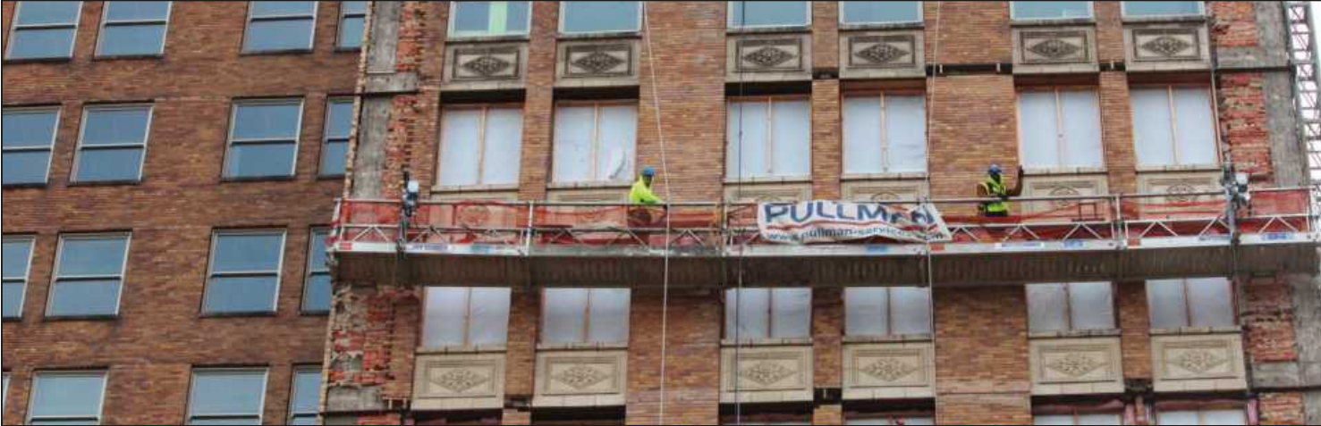
MAKING REPAIRS to the north side of the Residences @ 150 Bagley project in Detroit are masons John Gramlich and Phil Johnson. The Bricklayers and Allied Craftworkers Local 2 members are employed by Pullman Services
